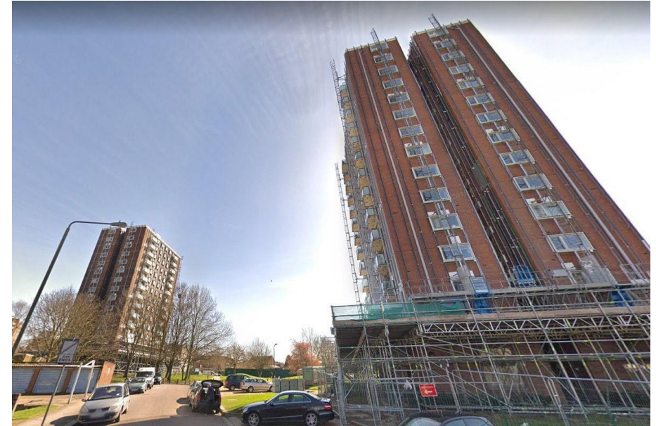
Many London local authorities have to invest in building safety improvements for their own stock (Picture above: the Granville Road tower blocks in Childs Hill during re-cladding, Source: Google)
